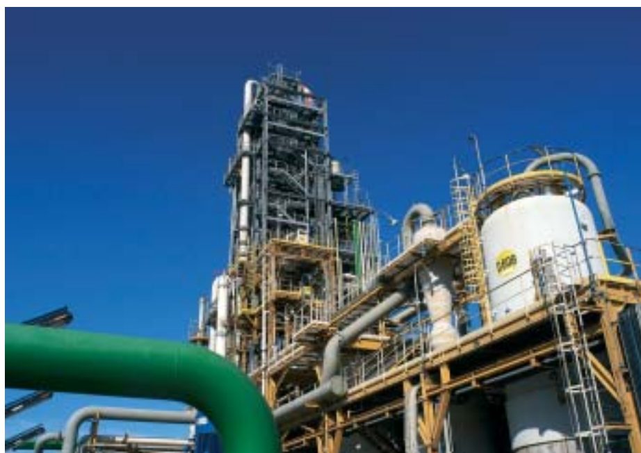
Basell Spherizone process plant in Brindisi, Italy. Spherizone is the latest generation Basell polypropylene technology.
