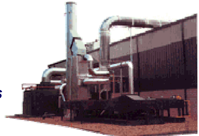
Solvent Recovery System
