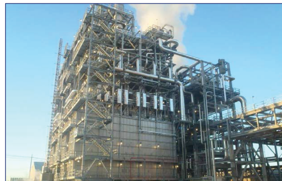
Completed La Porte Ethylene Furnace
